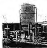
Waste water recycle plant for steel industry
