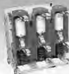
Vacuum Circuit Breaker (Rear View)
